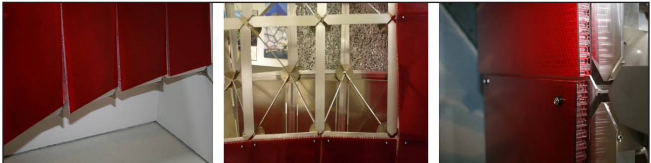
Fig. 3: Red Panelite composite polycarbonate panels used as cladding
